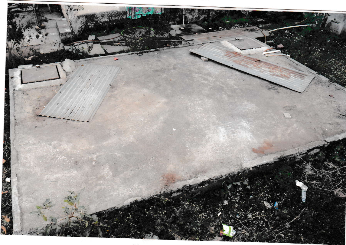
7.1.4 Water Conservation Facilities .
