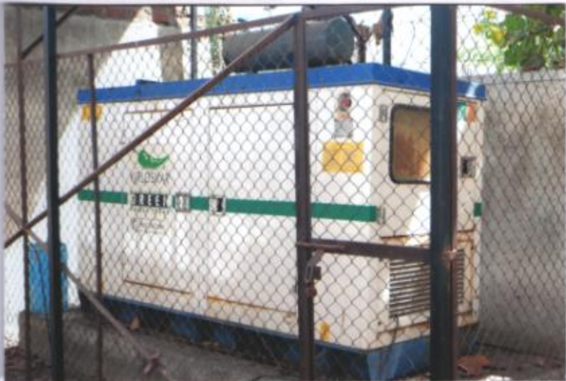
Battery Back-up [Inverter]
