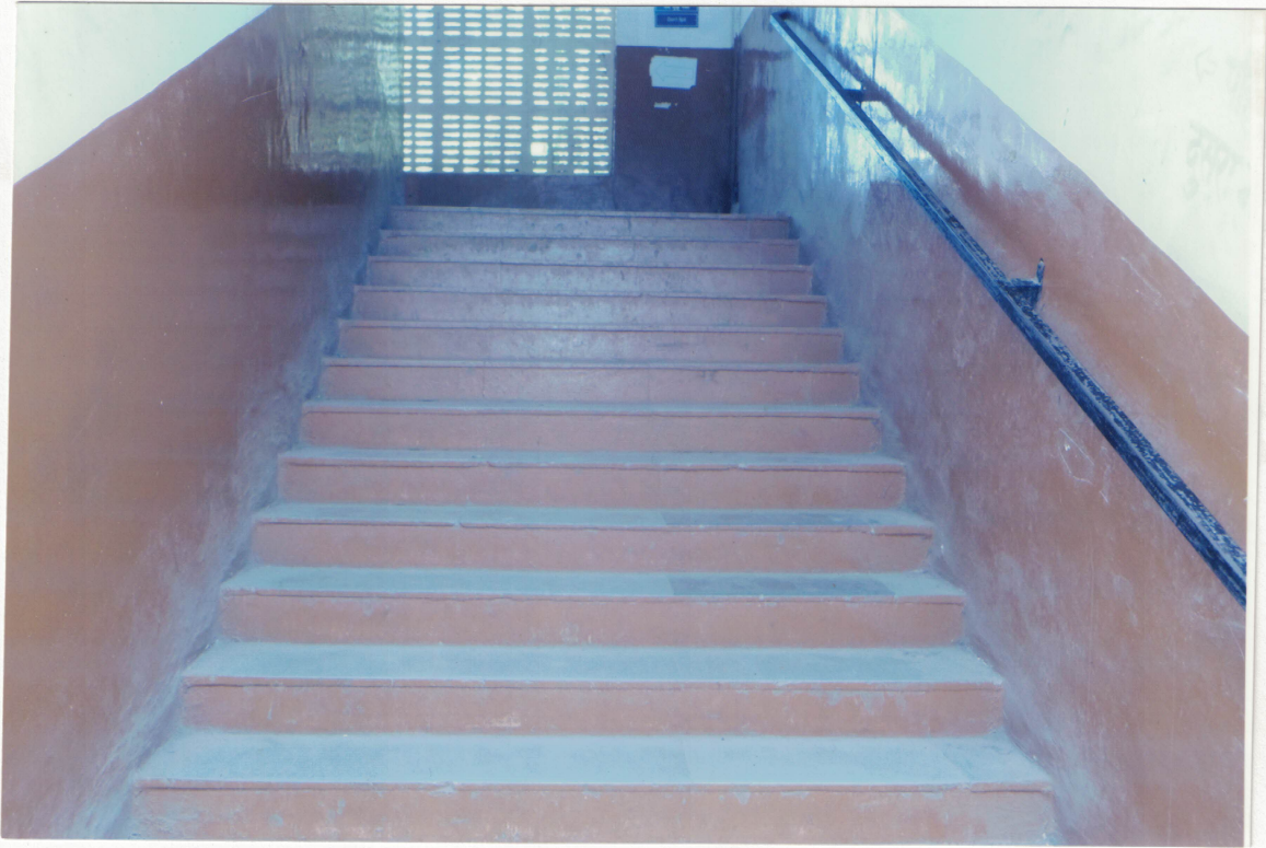
7.1.7 Railing for Disabled Students
