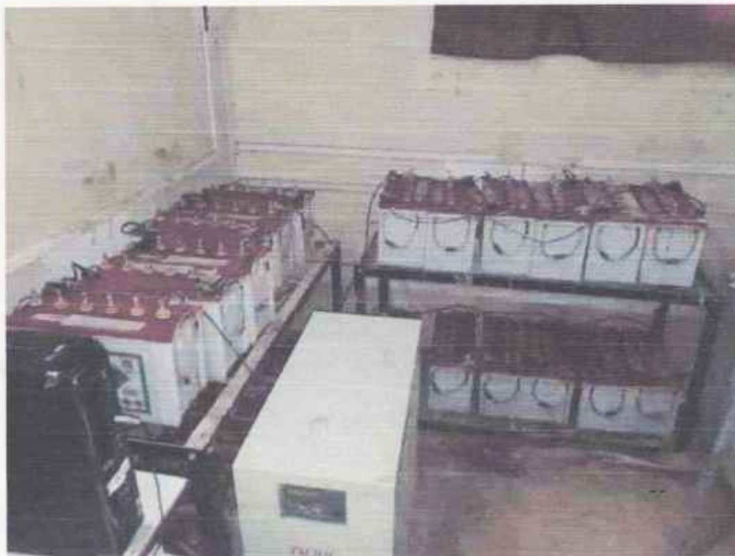
Batteries installed in the Computer Lab in the college
