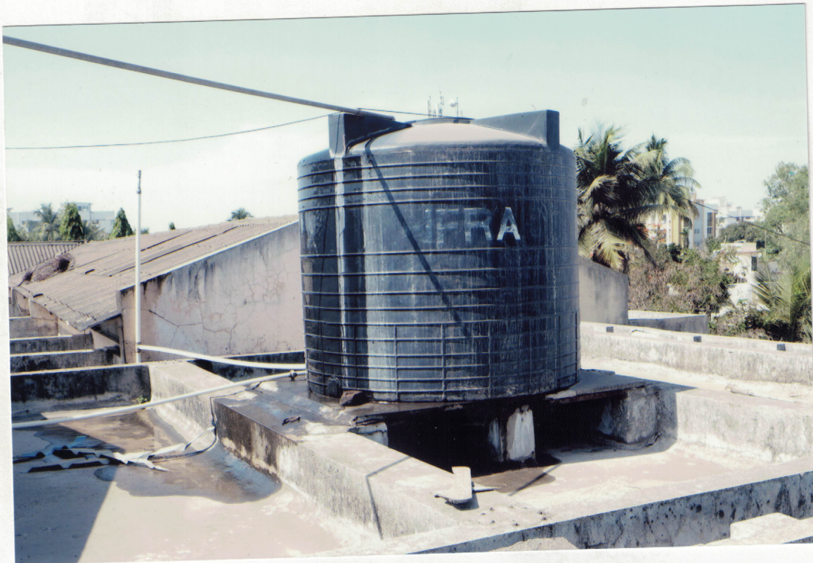
7.1.4 Water Conservation Facilities
