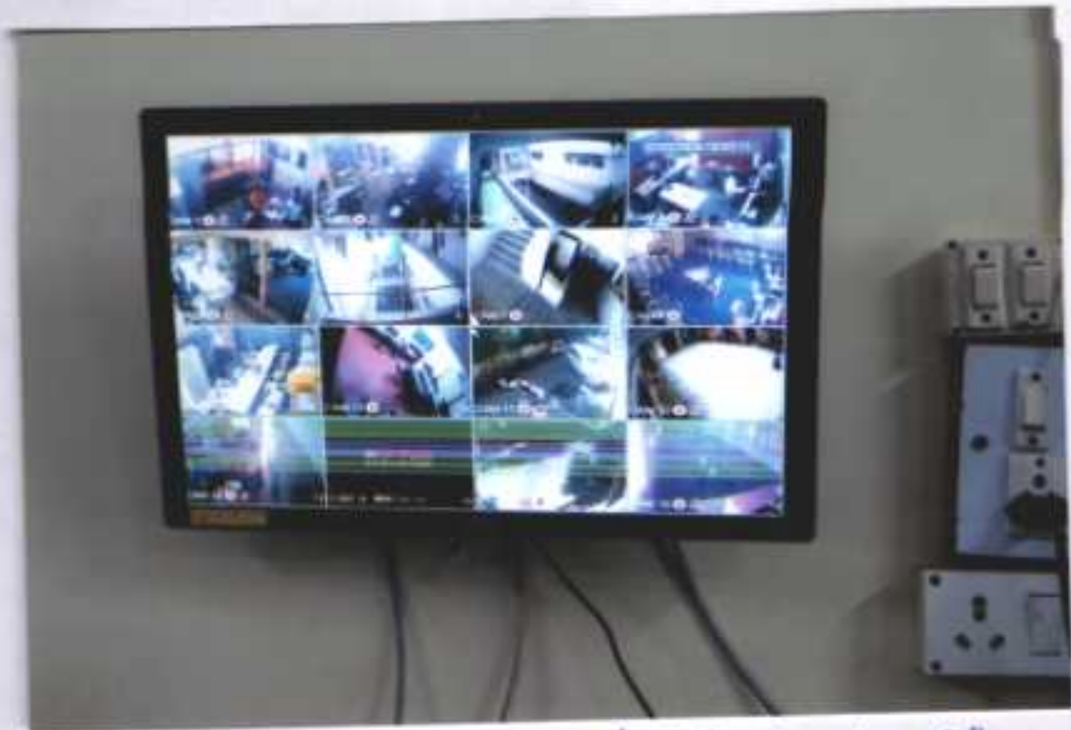
7.1.1 CCTV Cameras installed in the College
